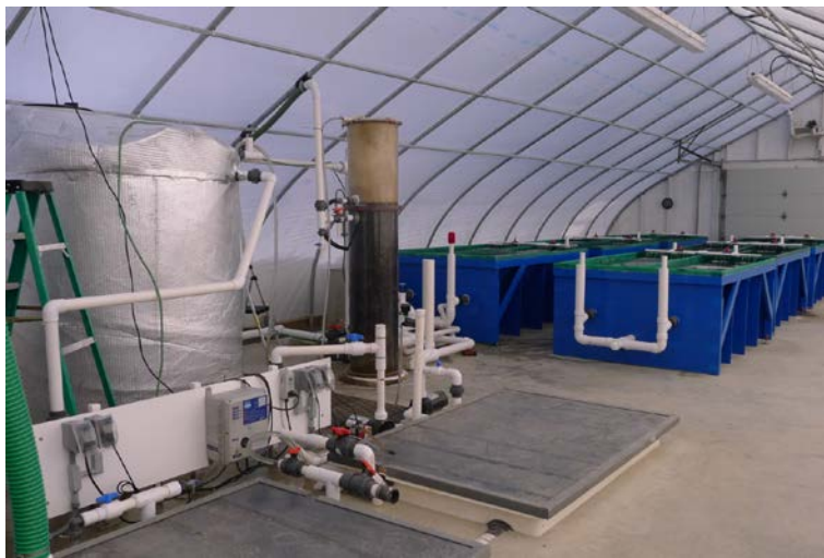
Figure 2: Urchin grow out system built for NRAC project.
